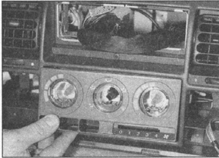
28.23 Pull the control knobs off the blower motor switch and heater controls, then undo the retaining screws and remove the front plate
